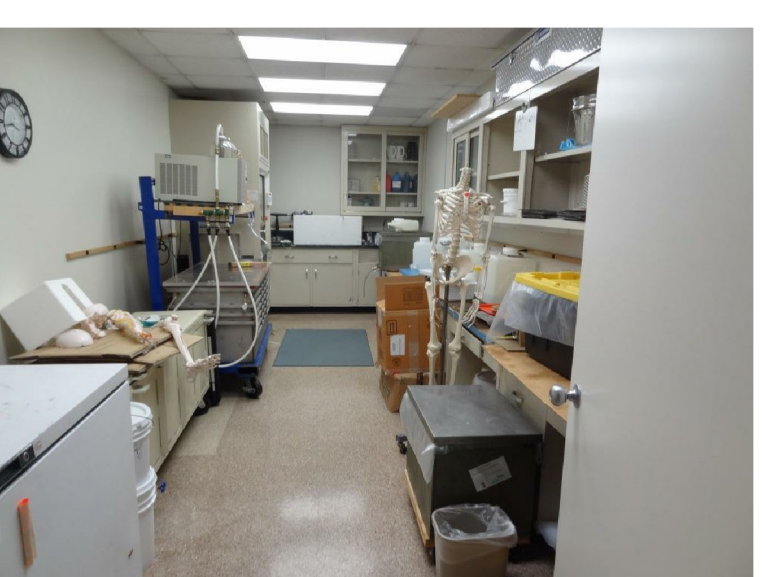
PHOTO #3 - ACM FLOOR TILE AND MASTIC IN ROOM 2065.
