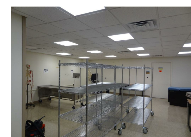
PHOTO #1 - ACM FLOOR TILE AND MASTIC IN ROOM 2063.
